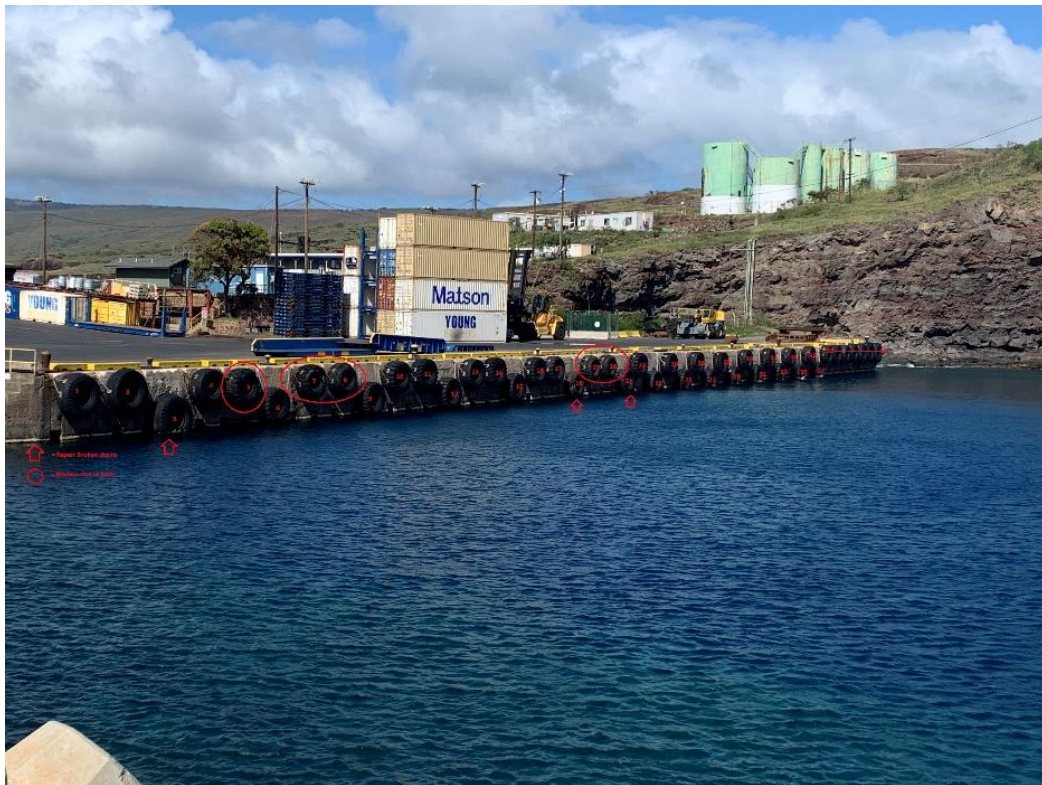
Photo 4: View of the five (5) tire fenders to be replaced along with chains and new shackles.
